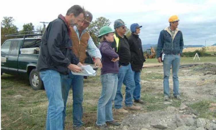
Dave Webb and Shasta Valley RCD staff touring the construction site with Siskiyou County Supervisor Jim Cook.
