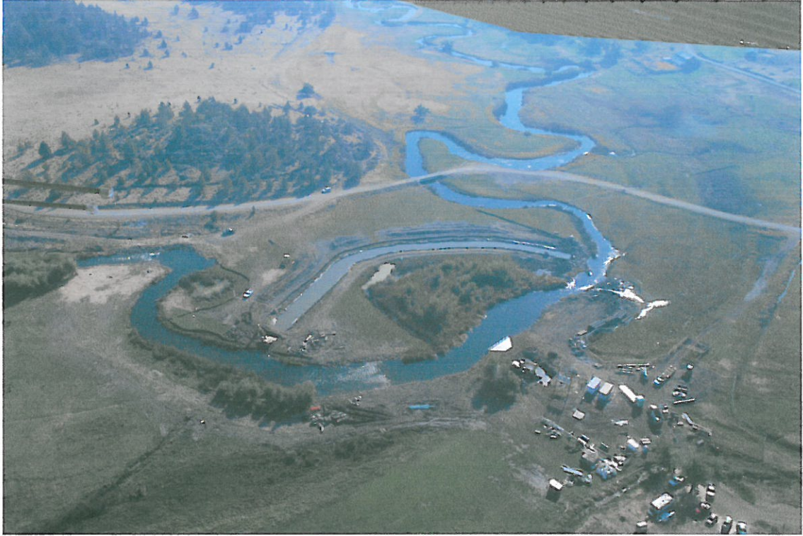
CDFG fly over of the project site. Photo showing the river back in its channel and the temporary bypass channel prior to backfilling.
